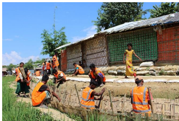
Refugee men engaging in a cash-for-work activity involving the building of sand bunds and staircases
